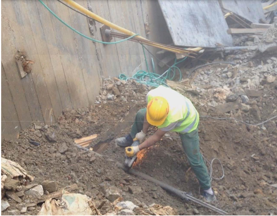
Figure 9: Cutting the soil anchor to the required length to be used as tendon
